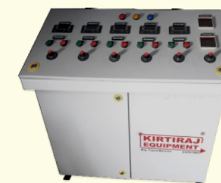
Motor Control Panel
